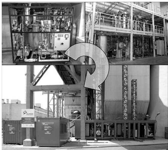
Fig. 1. Carbon Capture process scale up. Plants used during research: laboratory – 5 m 3 /h (upper left), research plant – 20–100 m 3 /h (upper right), pilot plant 200 m 3 /h (bottom)
