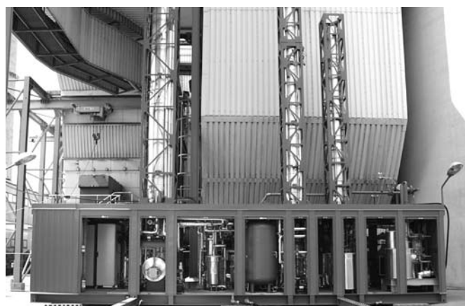
Photo 1. Technology Unit during the commissioning
