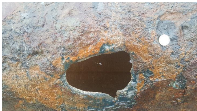
Fig. 4. Corrosion damage of water pipe as a result of stray currents
