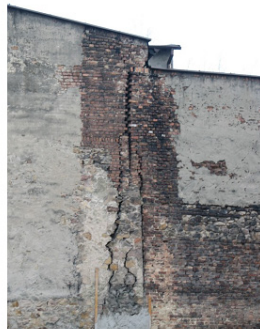
Figure 2. Multi-family house – a cracked supporting wall, in the area of intensive mining exploitation. Source: www.google.pl
