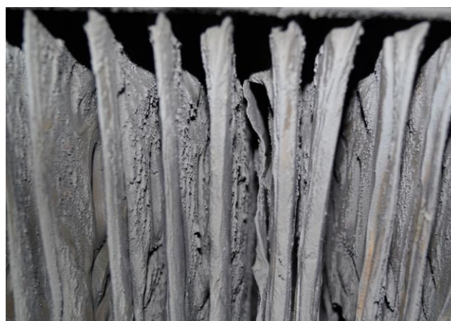
Fig. 5. Recuperator contaminated by overspray sediments
