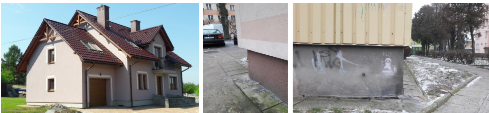
Fig. 6. Façade after thermal insulation creates contour greater than outline of building's ground floor (phot. M. Buško)
