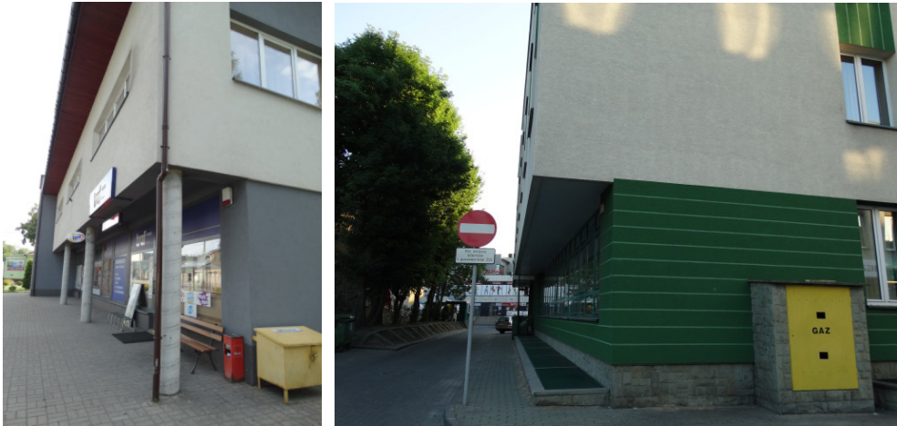
Fig. 8. Buildings with overhangs: supported and not supported by pillars (phot. M. Buško)
