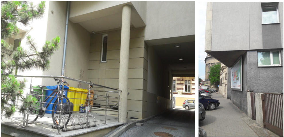
Fig. 7. Overhang of building supported by pillar and overhang not supported by pillar (phot. M. Buško)
