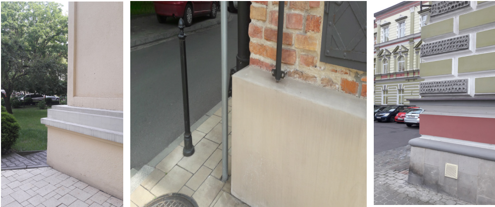
Fig. 5. Foundation wall creates contour larger than vertical projection of walls of higher story (phot. M. Buško)
