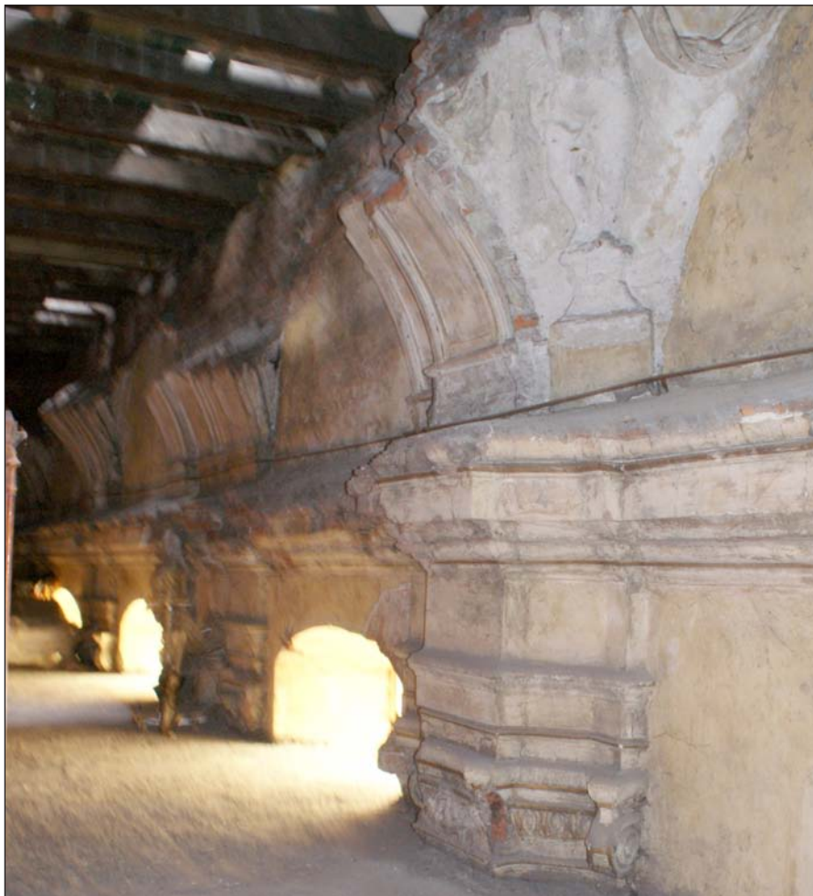
116. Remains of Baroque decoration of the nave of St Clare's Church above the reinforced concrete ceiling (2014); photo: E.G.
